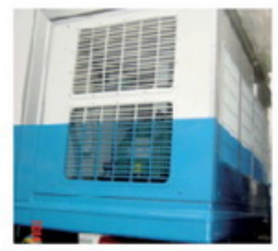
Condensing unit Cabin for easy maintenance access
